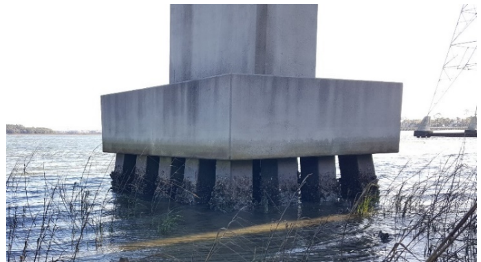
Oysters on existing bridge structures in Skull Creek. (Photo by Three Oaks Engineering)
